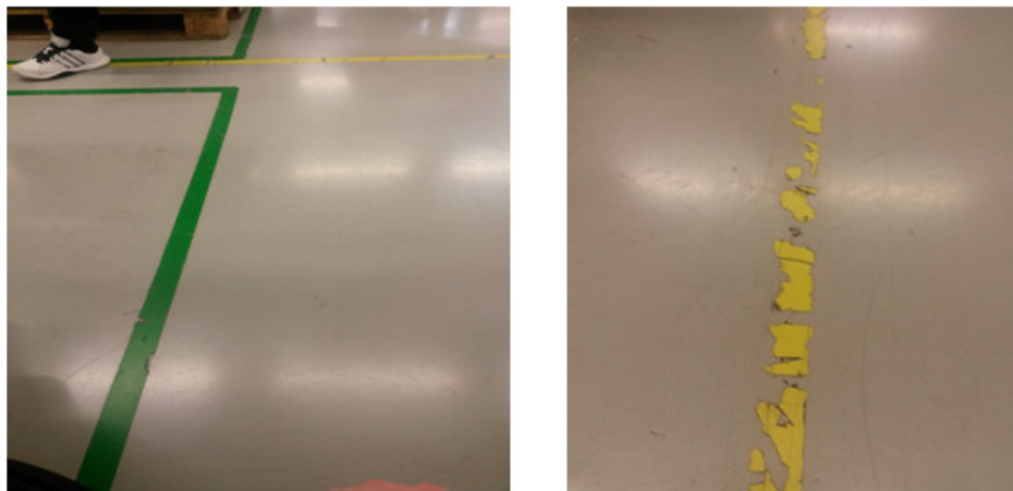
Fig. 2. Conforming and non conforming aisle markings
